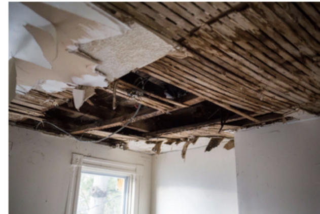
A dilapidated home in Baltimore. Al Drago/The New York Times
